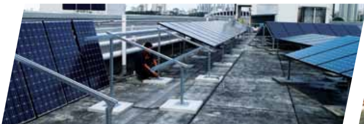
SINGAPORE POLYTECHNIC System Size 10.08 kWp
