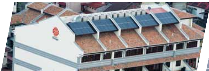
HOTEL PENAGA, PENANG, MALAYSIA System Size 20.79 kWp
